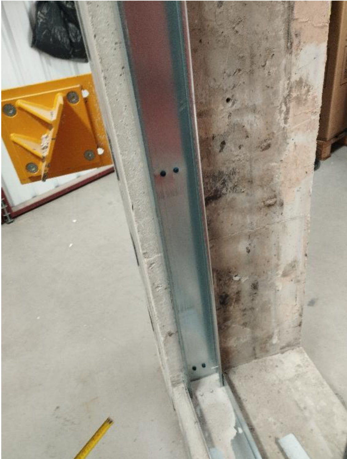
Photograph 2 – Base track fixed into the frame
