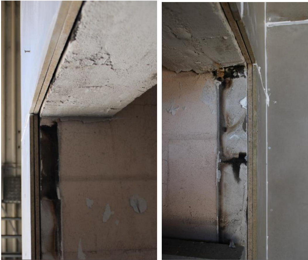
Figure 7. Double layer of sheathing board at combustion chamber surround.
