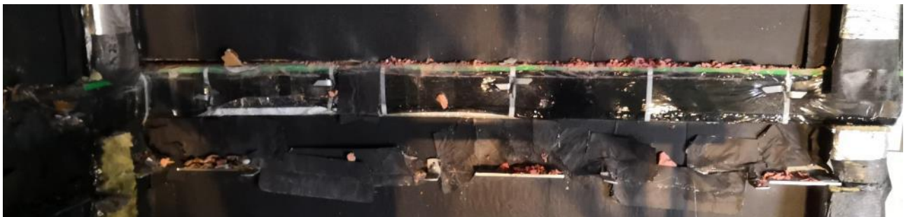
Figure 4.21. Post-examination damage. Photo of the bottom horizontal fire barrier installed on the wing face. In-place and without been activated.
