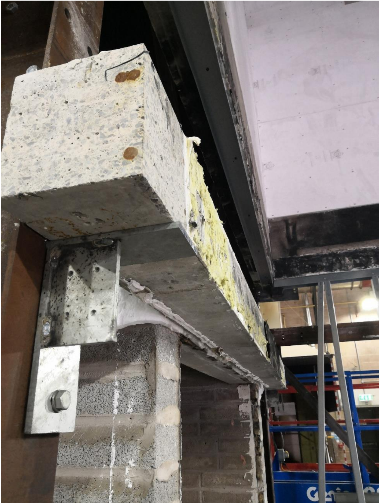
Figure 4.2. Installation of concrete lintel in front of combustion chamber's lintel on the main face during construction.
