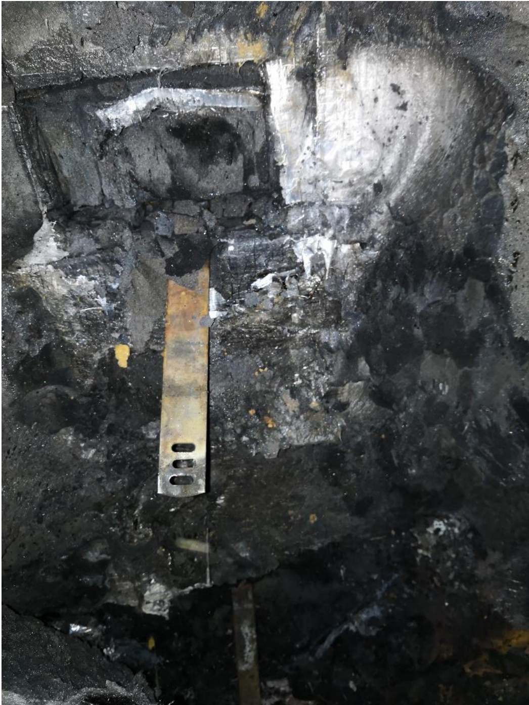
Figure 4.23. Post-examination damage. Photo of one bracket located just above the combustion chamber. No damage except discoloration observed.
