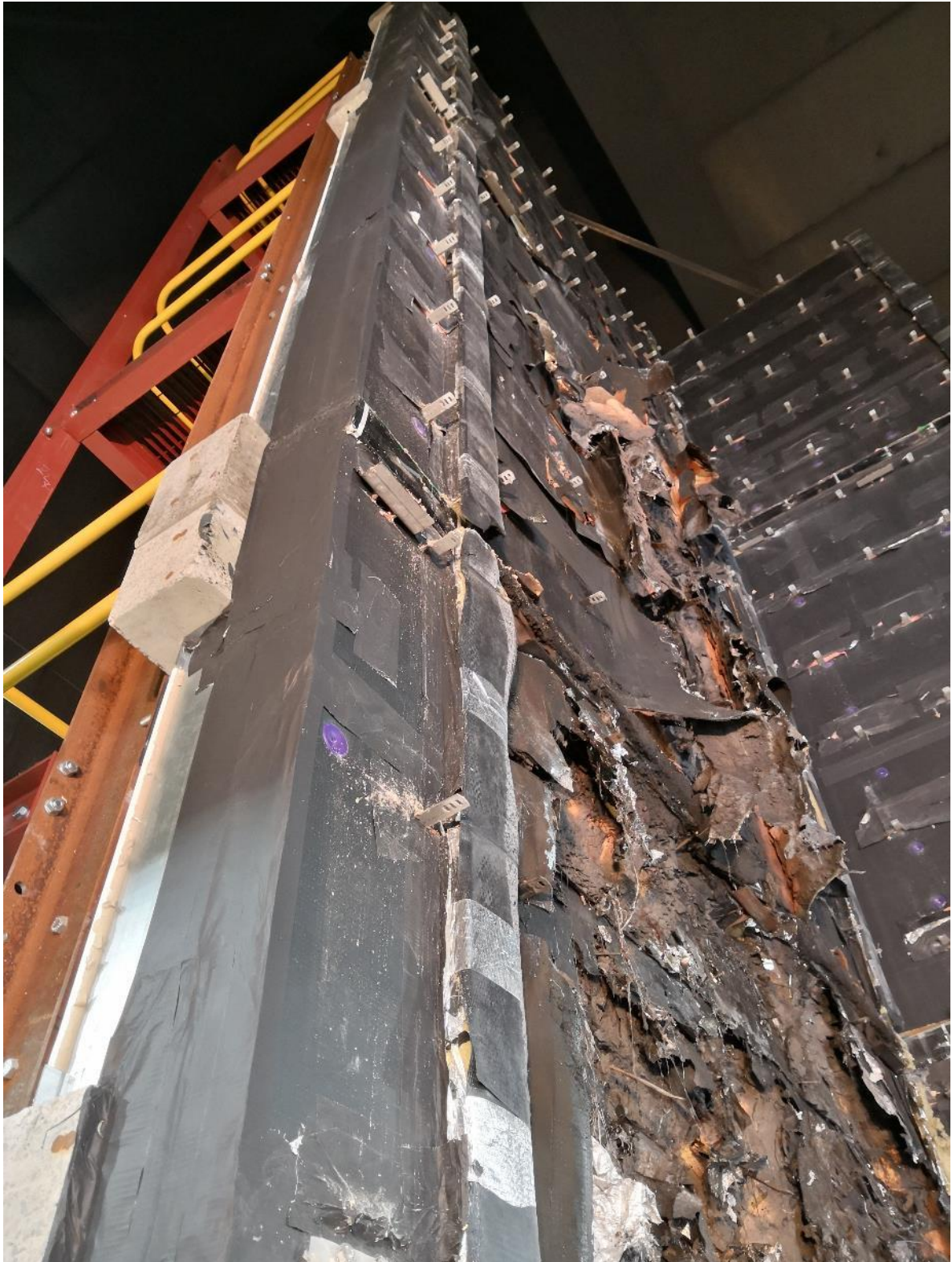
Figure 4.19. Post-examination damage. Vertical fire stop barrier located on the left-hand side edge of the system's main face. No damage observed; in-place and intact.
