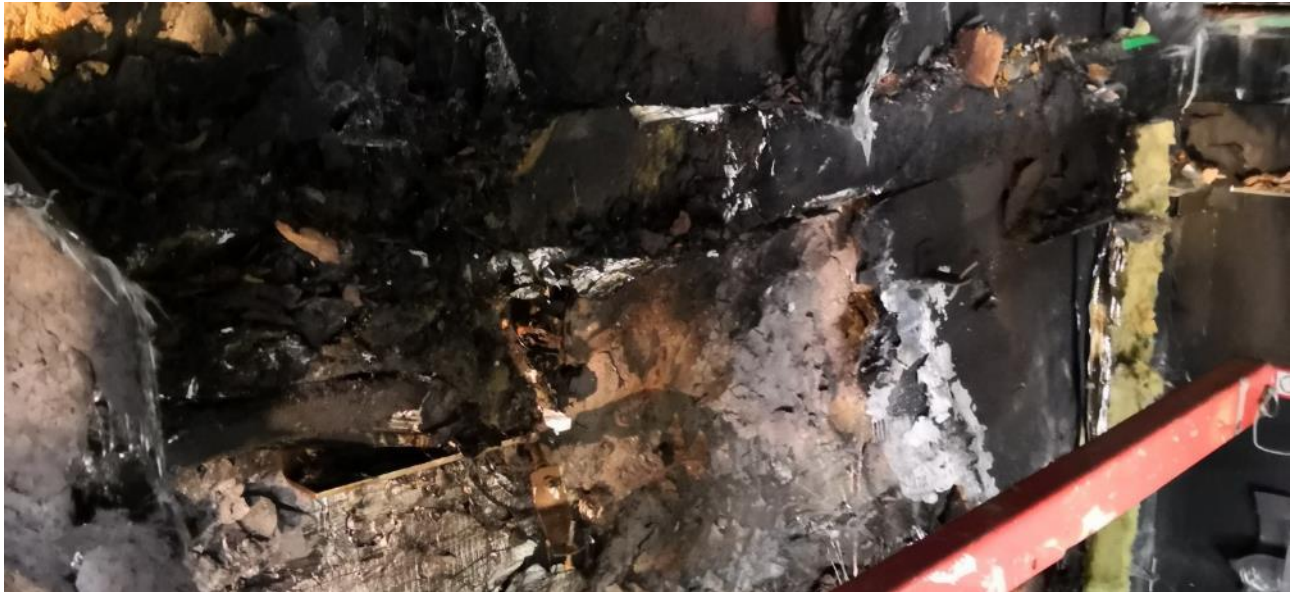
Figure 4.20. Post-examination damage. Photo of the bottom horizontal fire barrier installed on the main face. Fully activated and partially detached (especially above the chamber).
