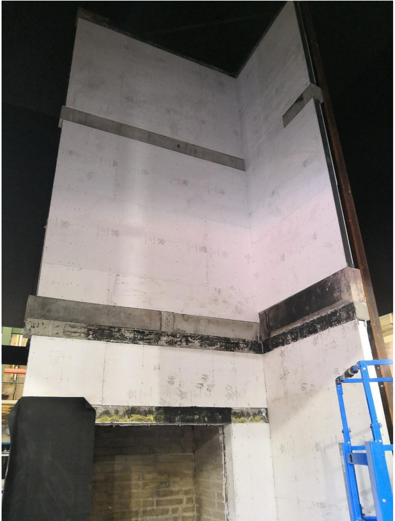
Figure 4.4. View after completing sheathing board layer mounting during construction. Start of waterproof membrane installation.
