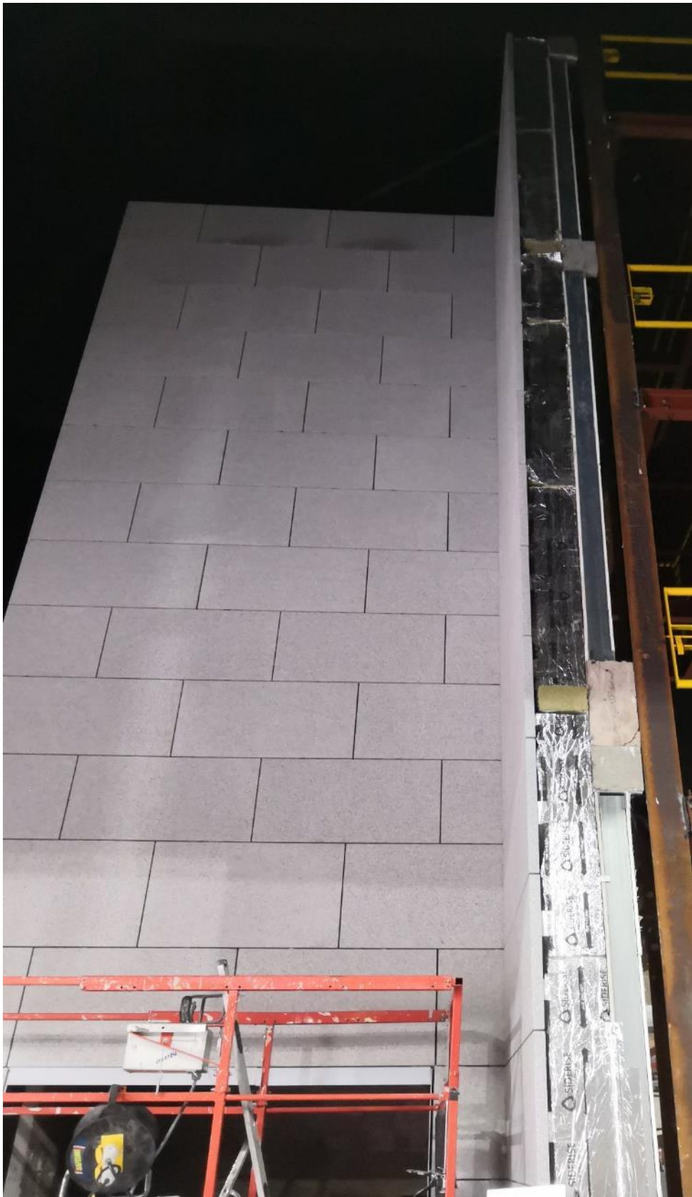
Figure 4.10. Front view of the finished main face of the system just before the test.
