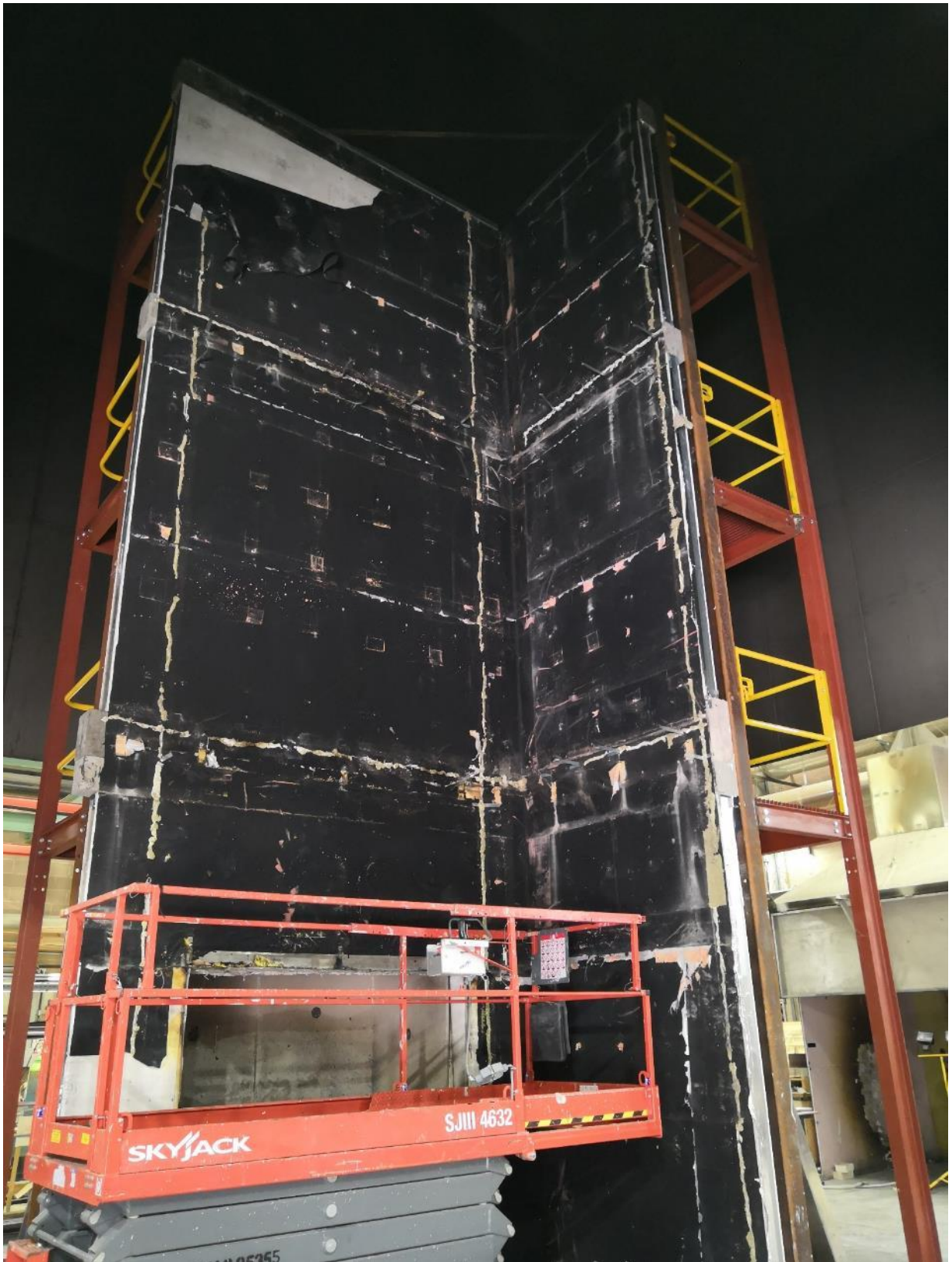
Figure 4.24. Post-examination damage. Waterproof membrane intact and in place after removing insulation layer from system.
