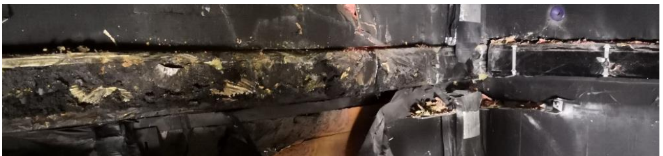
Figure 4.22. Post-examination damage. Photo of the middle horizontal fire barrier installed on both faces. Partially activated on the main face but in-place; not activated or detached on the wing face.
