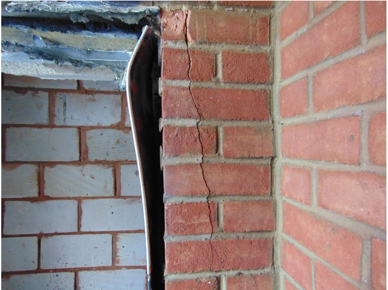
Figure 22. Cracking local to inside edge of combustion chamber opening.
