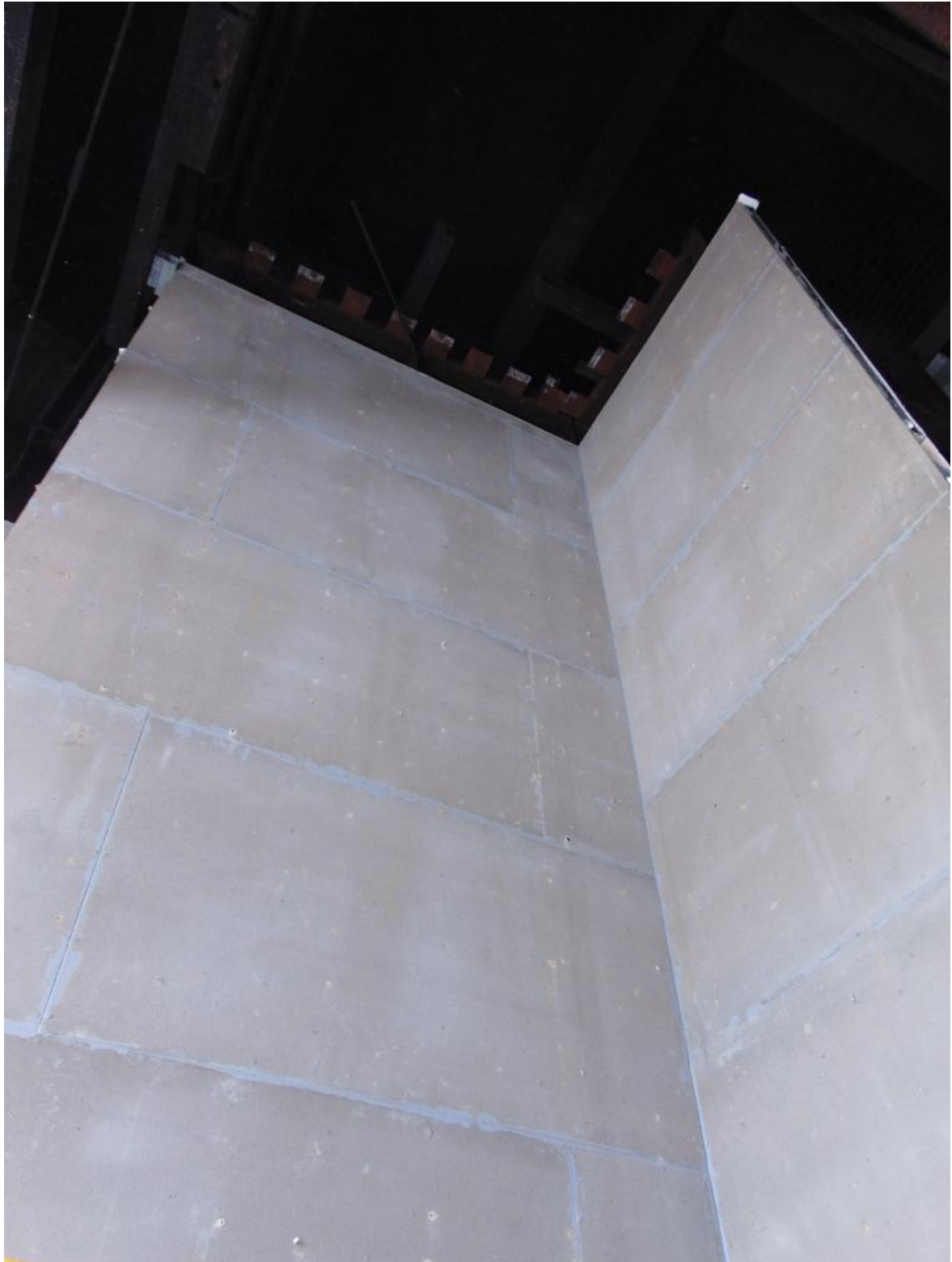
Figure 31. Cement particle board from a height of approximately 2000mm above the top of the combustion chamber to the top of the cladding system.
