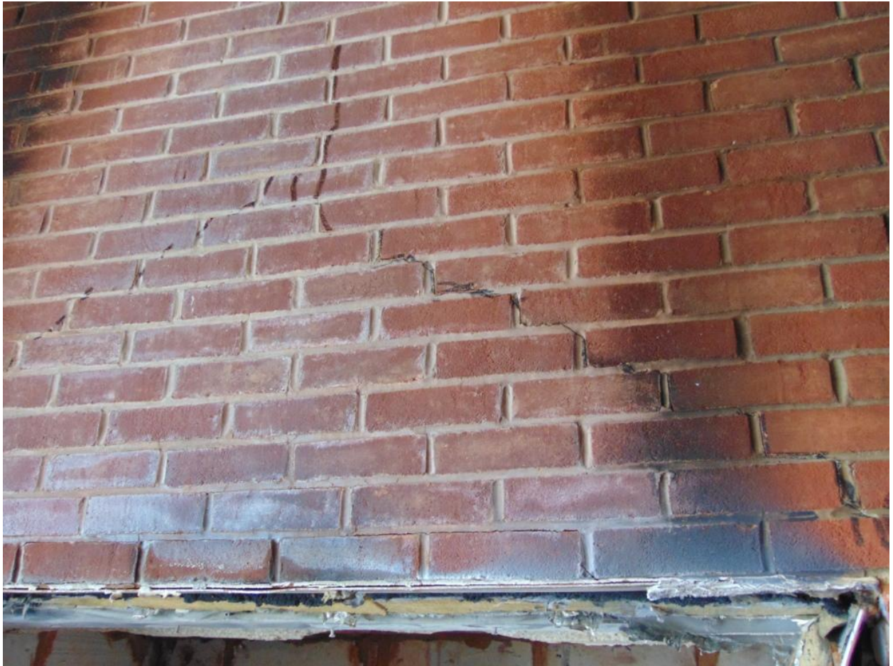
Figure 24. Cracking in brick façade above combustion chamber.
