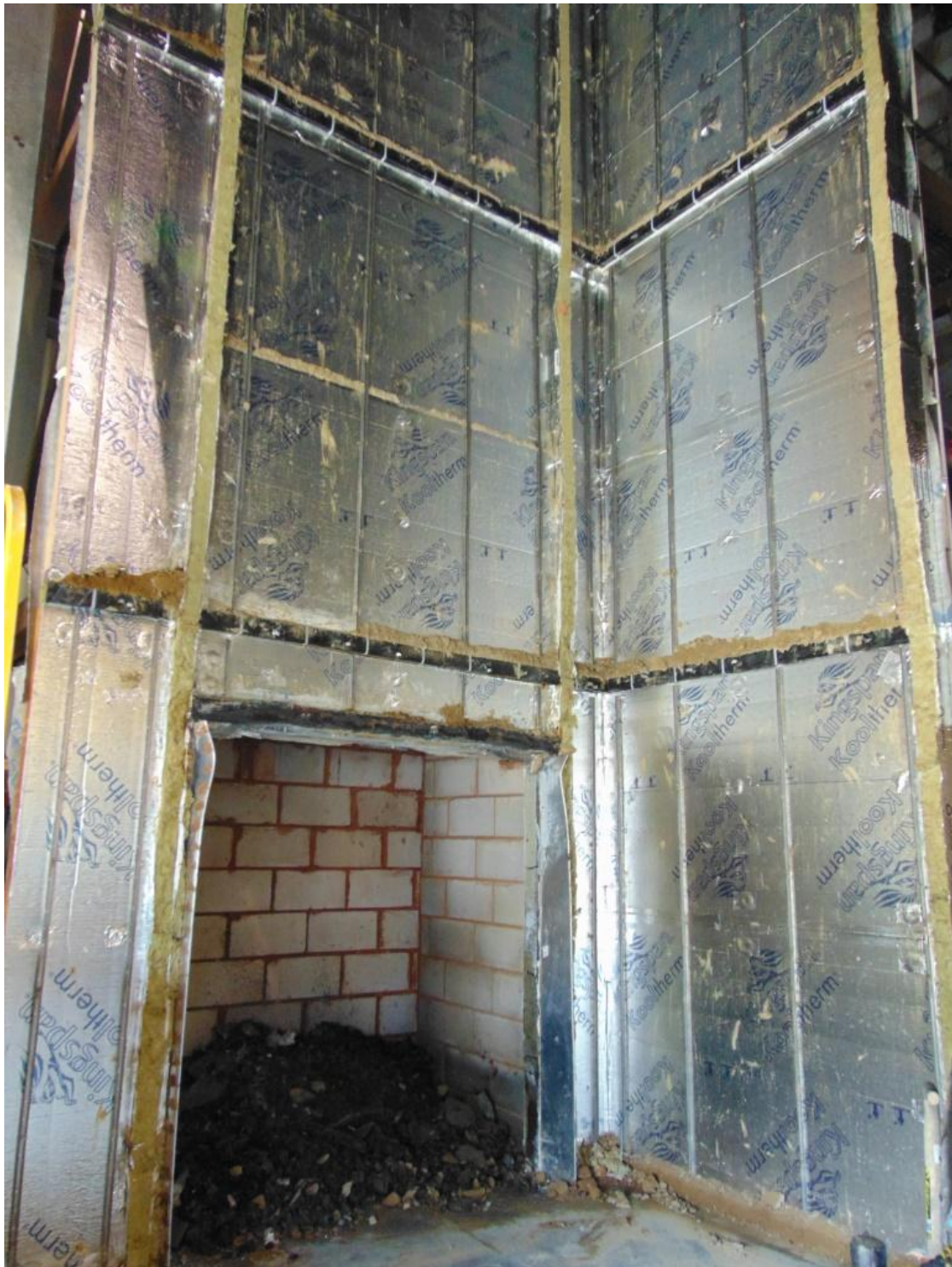
Figure 26. Photograph of insulation from ground to a height of third row horizontal cavity barrier.
