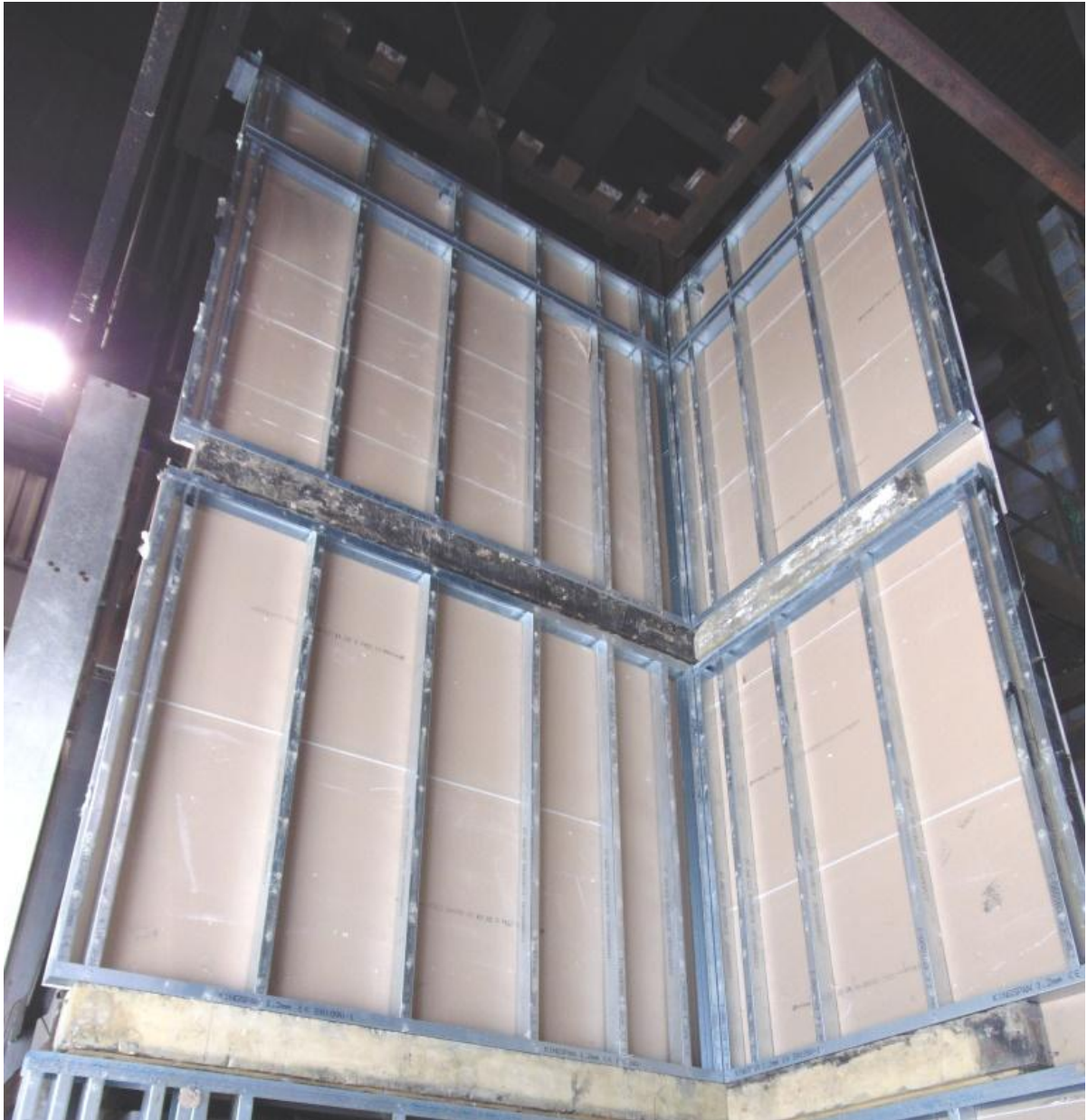
Figure 33. Lightweight steel framework partition from first row floor slabs to top of cladding system.
