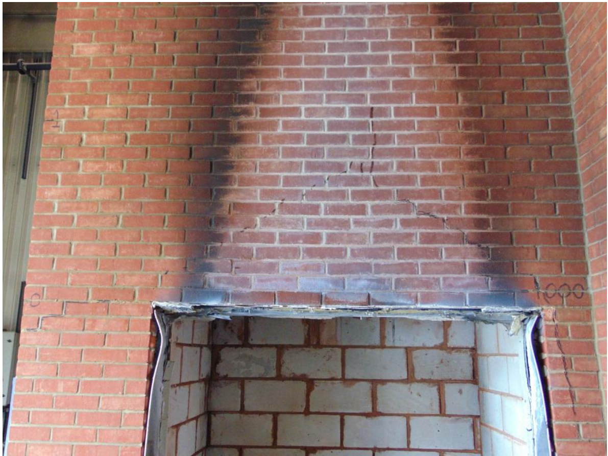
Figure 23. Cracking in brick façade.
