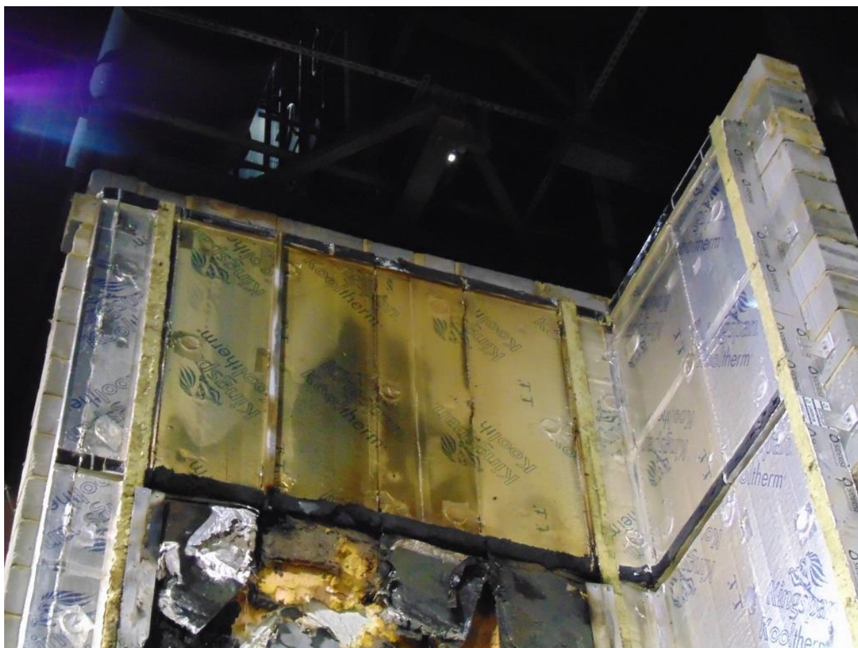
Figure 19. Post-test photo between third and fourth row Siderise RH25G 90/30 horizontal open state cavity barriers.
