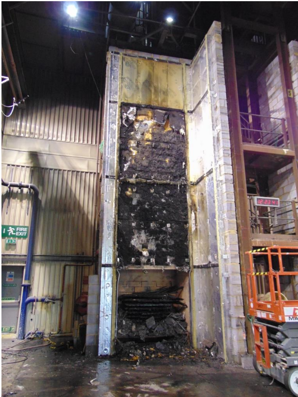
Figure 16. Full-height photograph of system following removal of ACM panels and aluminium rail substructure.
