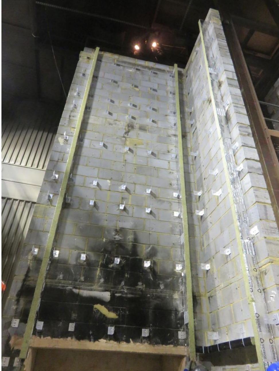
Figure 4. 'L'-shaped aluminium brackets installed with Siderise RSV 90/30 vertical cavity barriers fitted on main and wing wall.
