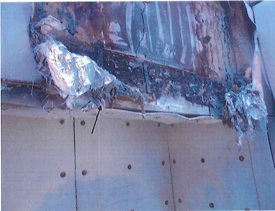
DLP C2753J/0015 Cavity barrier above the combustion chamber
