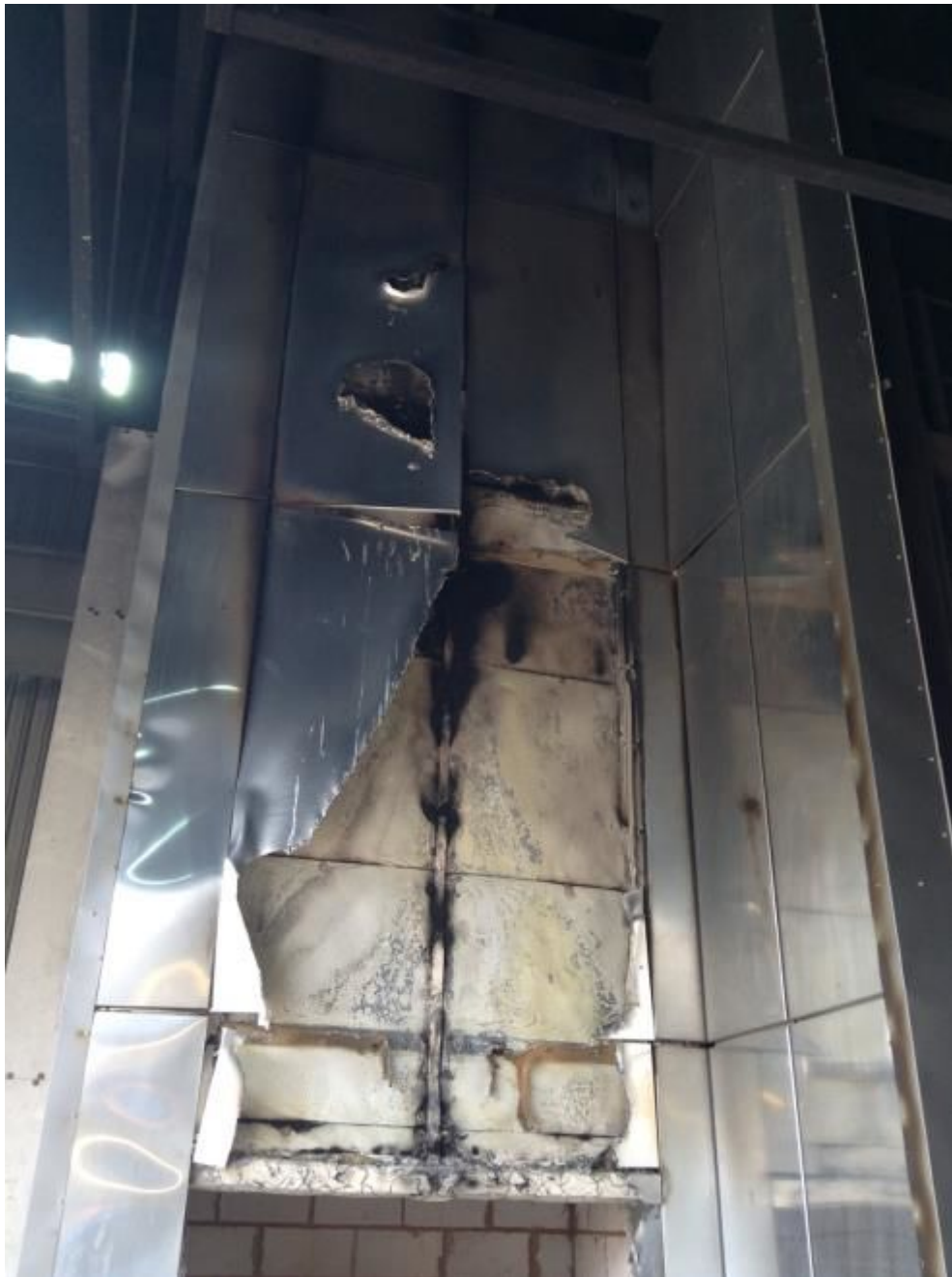
Figure 18. Photograph showing the condition of the cladding system post-test (Decorative Layer Full height).
