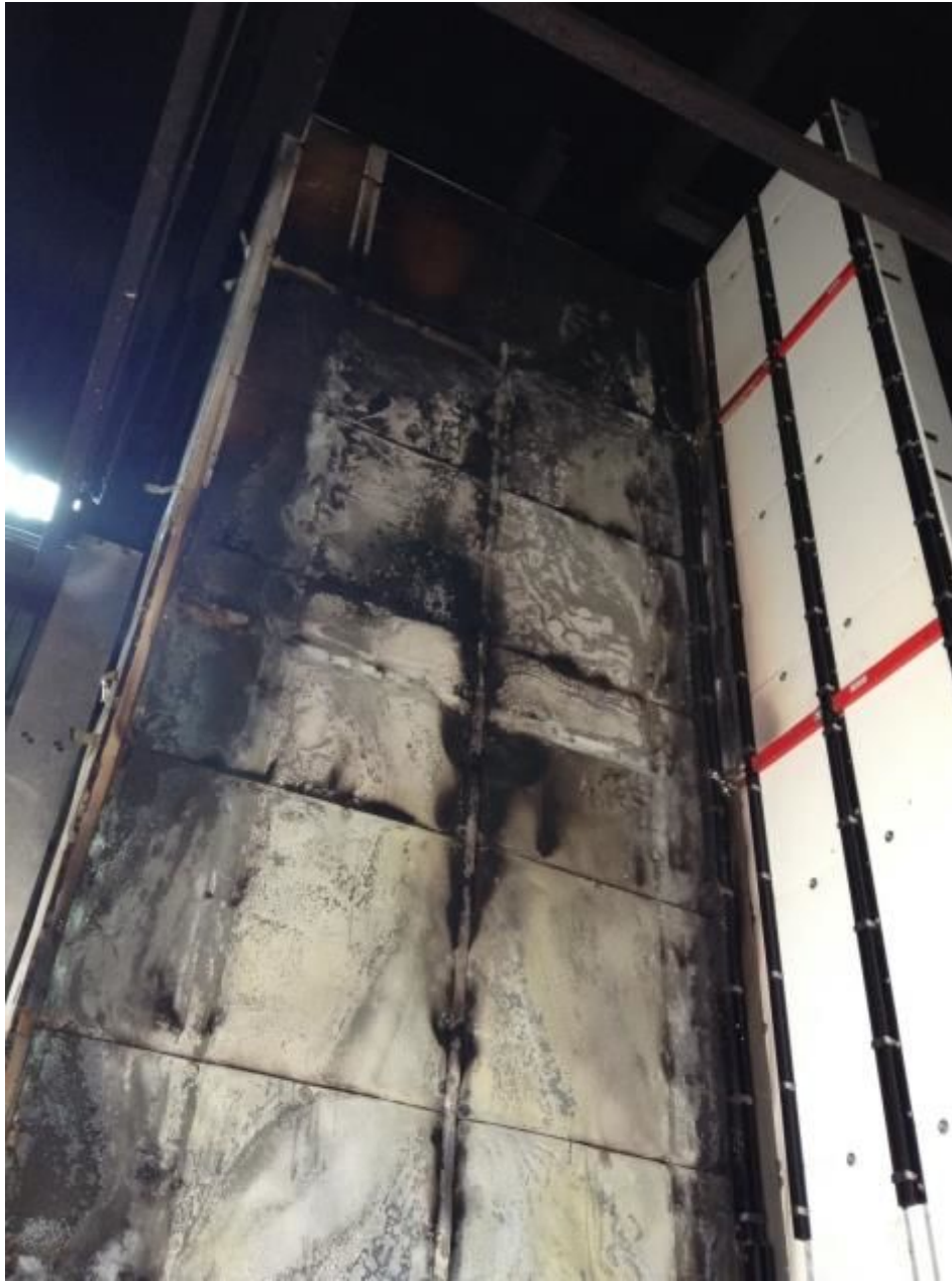
Figure 20. Photograph showing the condition of the cladding system post-test (Insulation Layer Full height).
